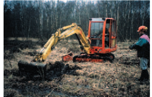
After felling one ha of birch in the Landes de Versigny Reserve, the Conservatoire des Sites Naturels de Picardie began mechanical turf stripping (removal of upper layers of peat) in order to restore the young stages of the peat bog.
